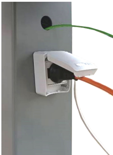
Fig. 20: Example of internal power socket
